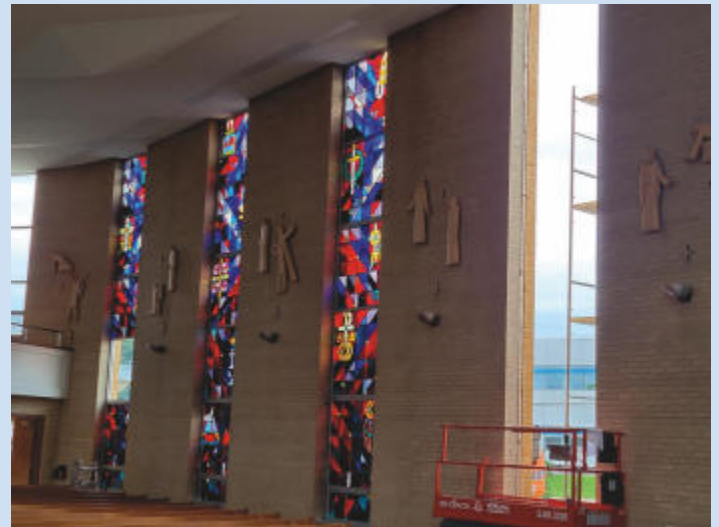
The stained glass installation began Aug. 23 and will take a few weeks.
