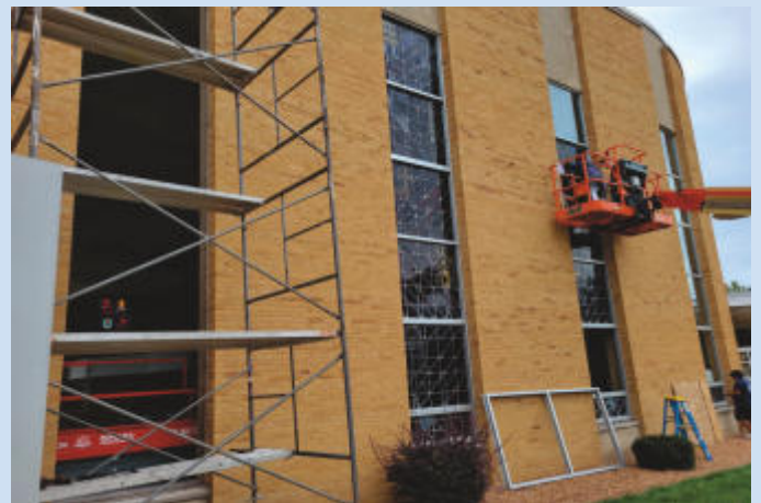
Process: original glass removed, old frame removed, new frame fitted, stained glass installed, clear protective glass installed, and frame caulked.
