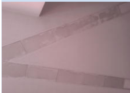
Ceiling grills hang in the diagonal lines which include the light panels.
